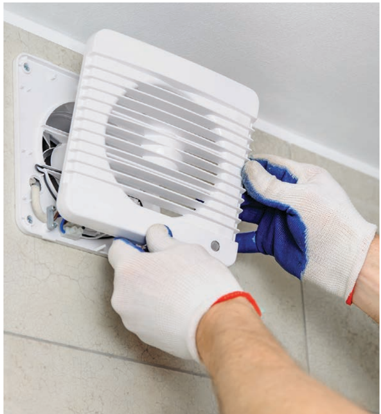
Installing ventilation can help get excess humidity out of your home, making it more comfortable and also reducing the possibility of water damage due to condensation.
