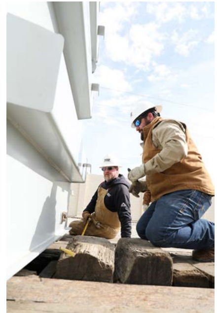
TVEC linemen Shane Bardin and Coin Pool prepare a new substation transformer for a crane lift to its permanent home in the new Tool substation.
