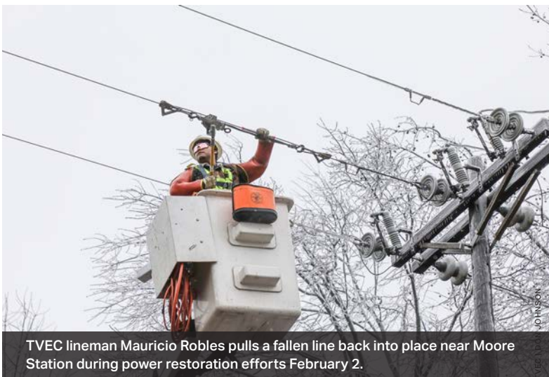
Line crews and tree trimmers worked in overlapping 16-hour shifts ensuring the power restoration work never stopped.
